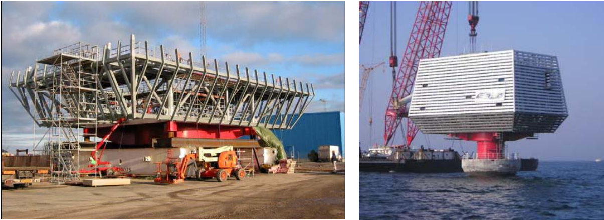
Figure 8-10: Construction and installation of the Nysted wind farm transformer station (Source: Bladt Industries A/S).
