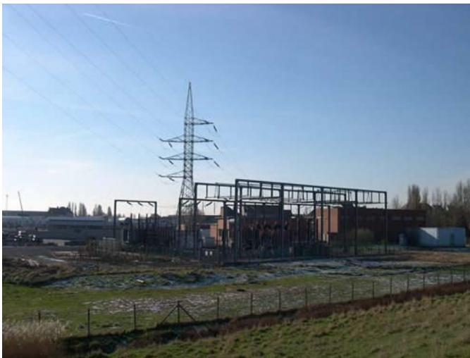
Figure 3-9: The grid connection point at the high voltage (150kV) substation at Slijkens in Bredene, Oostende.
