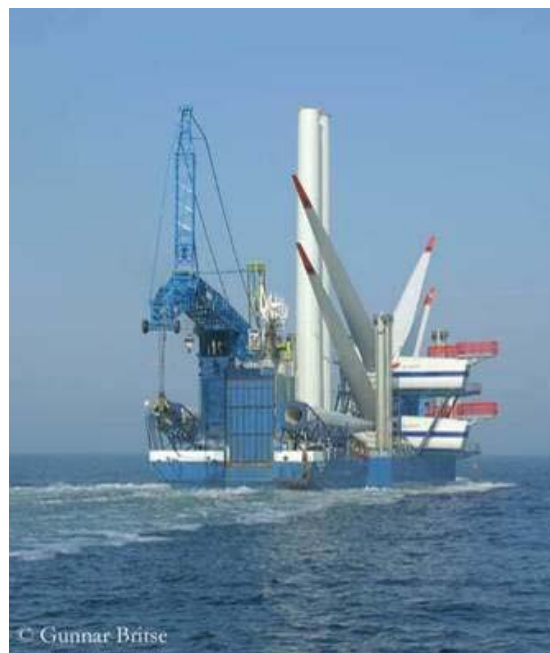
Figure 7-16: The crane vessel “Ocean Hanne” was used for turbine transport and installation (Source: Gunnar Britse).
