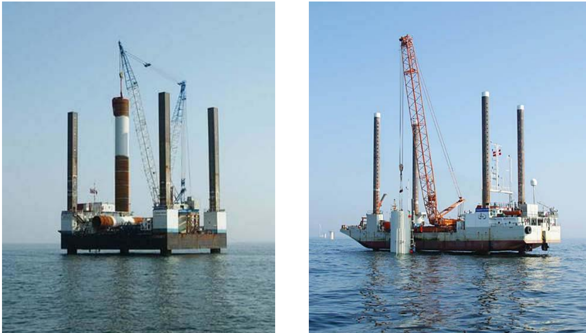
Figure 7-14: Pile driving (left) and installation of the transition piece (right) was carried out by jack-up platforms from Ballast Nedam (Source: Gunnar Britse).
