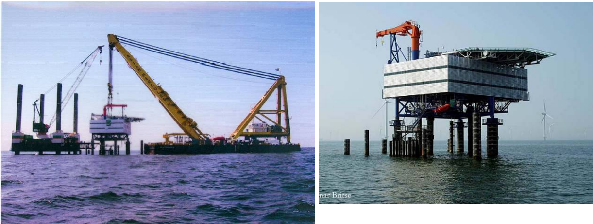
Figure 7-15: Left: “Asian Hercules” delivering the 1200-tonne substation (Source: ELTRA). Right: The ready installed 36 kV to 150 kV substation (Source: Gunnar Britse). The medium voltage cables from the turbines are connected to this substation.
